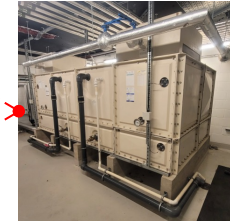
Cold Water Storage Tanks 2x
