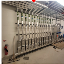
Flats – Stopcocks & Meters
