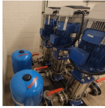
Booster Pumps Set
